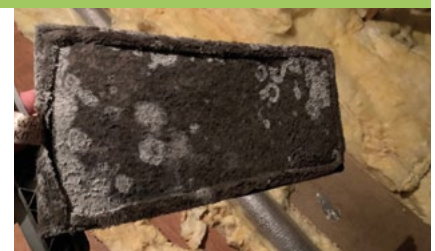
Six-year-old MVHR unit filter that had not been serviced. Clogged filters lead to higher operating costs and inhibit a system's ability to filter out particles such as dust and pollen
