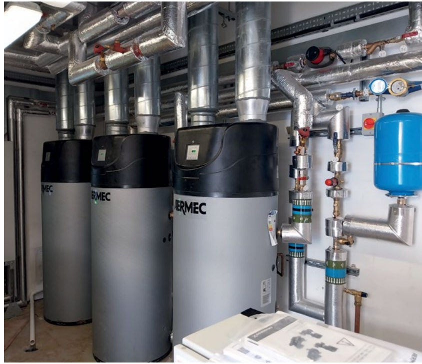
West Coventry Academy has air source heat pumps for heating and kitchen hot water
