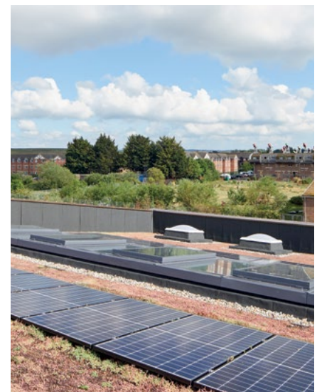
The 424m 2 of PV panels are designed to deliver 81kWp
