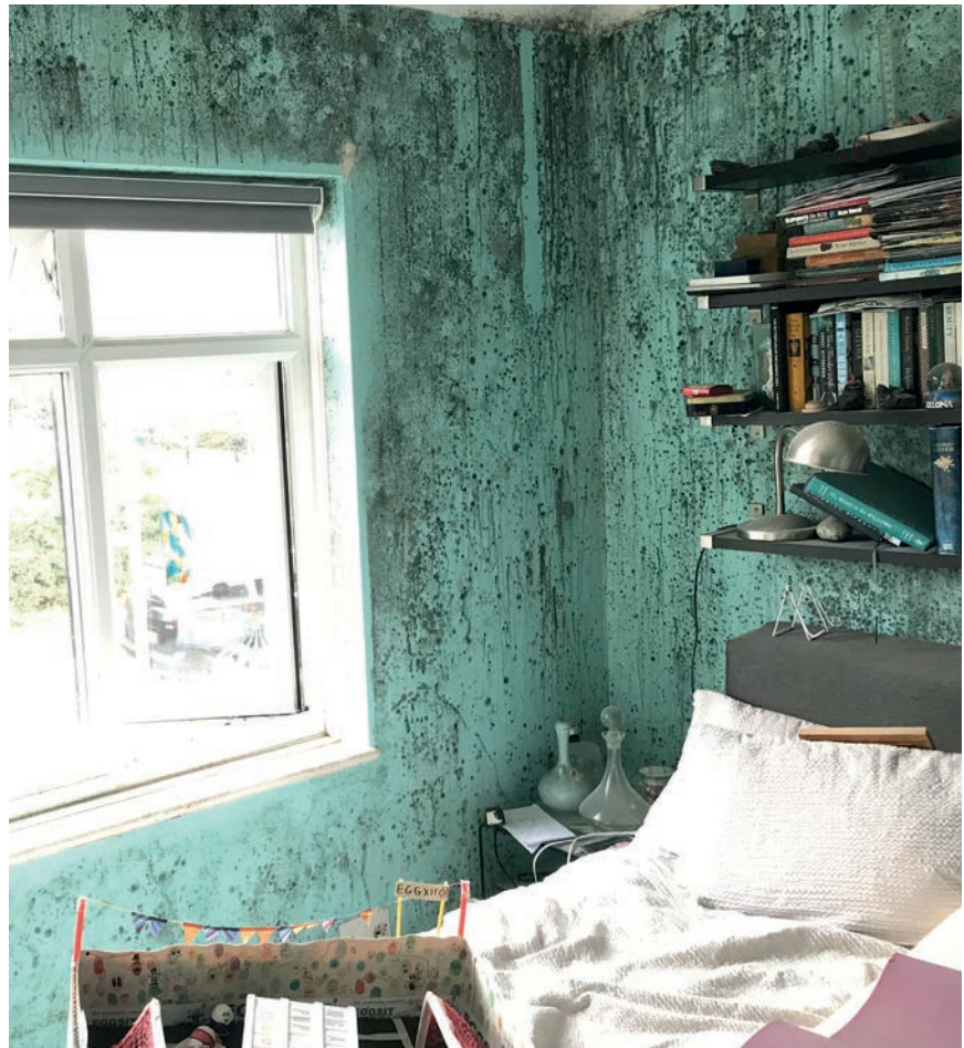
Figure 1: Extreme example of the consequences of poor ventilation in first-floor bedroom when room was closed up for 12 weeks during ground-floor building works in winter 2021-22. A trickle vent in the top corner had been previously plastered over (Photo source: Martin MacDonald)
