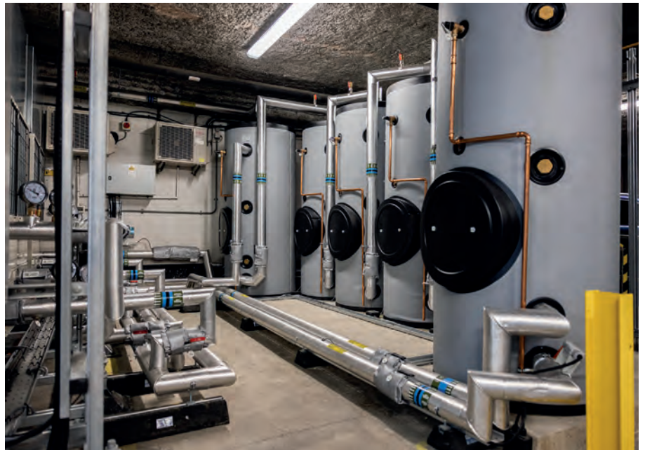
6000 litres of potable hot water satisfy the hotels peak demand
