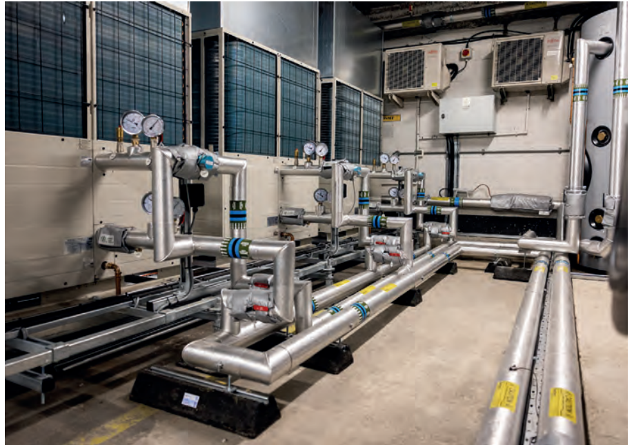
Three Q-ton modules designed and installed inside a plant room with sufficient air flow
