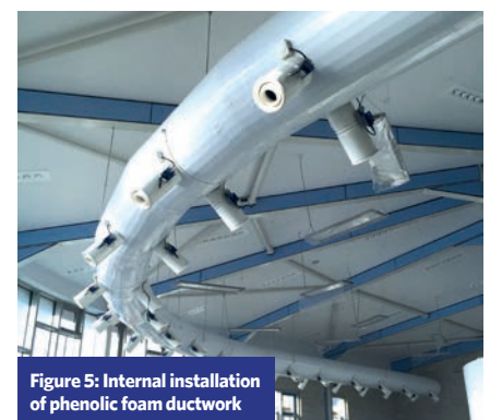
Figure 4: Weather-protected installation of a phenolic ductwork system on exposed roof. The weatherproof UV resistant laminate is tested up to 148°C
