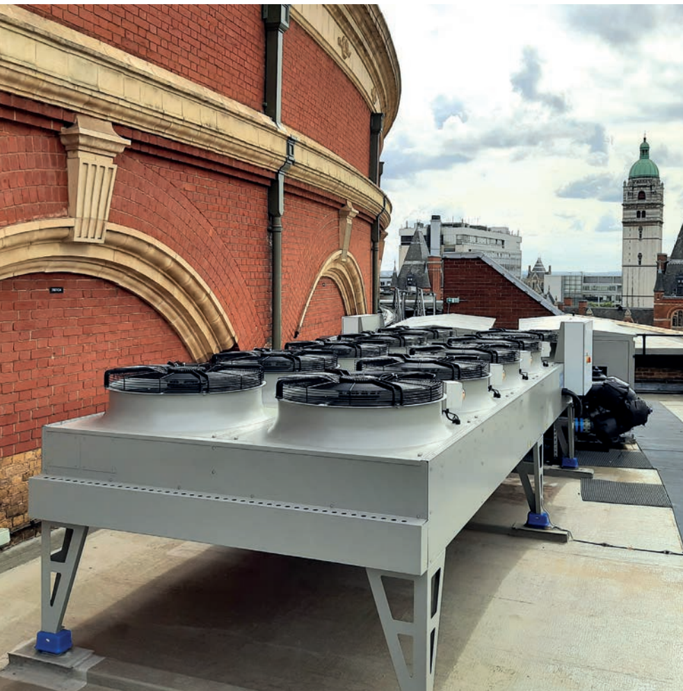
To minimise visual impact on the roof Loop Engineering specified flat-bed remote air-cooled condensers for heat rejection
