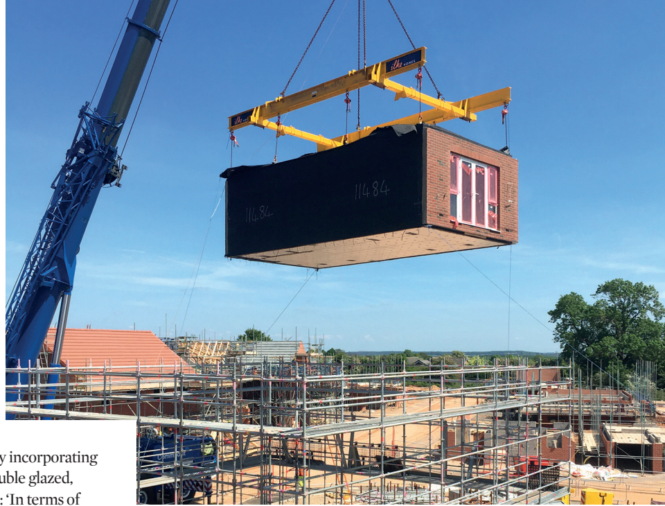
Factory-built modules arrive on site fully finished and ready to be craned into position
