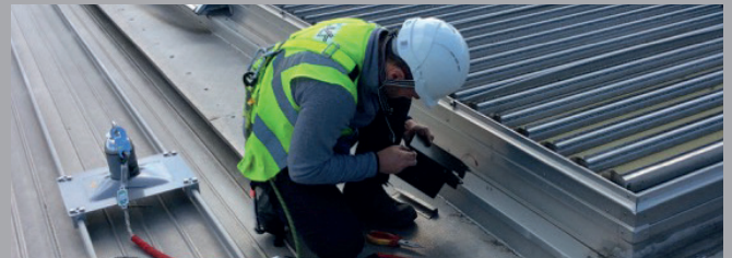
Product testing inspection underway, prior to the commissioning of a newly installed smoke control system.
